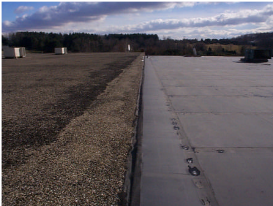
PHOTOGRAPH 14 Repairs along south side of roof and at membrane tie-in to adjacent EPDM roof membrane.
